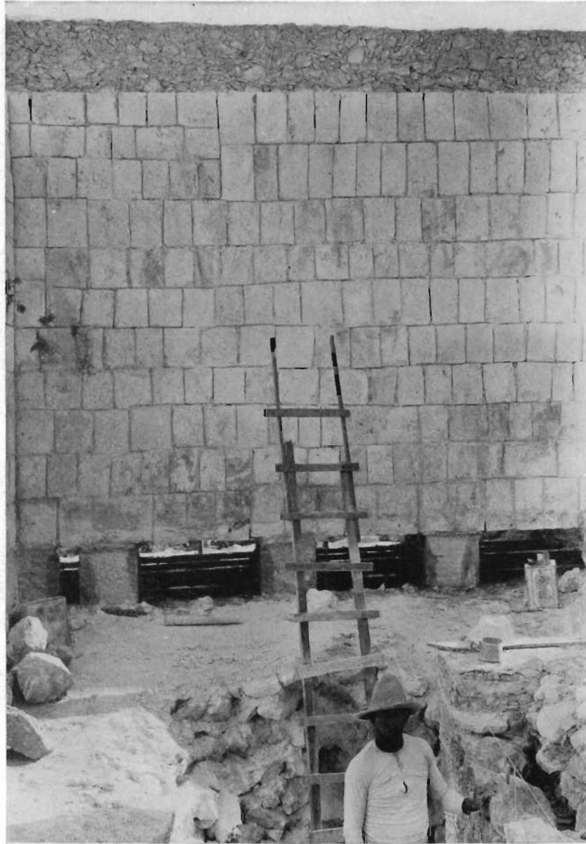
FIG. 91—NORTH WALL, I-BEAMS OF FOUNDATION IN PLACE, SEEN FROM INTERIOR OF TEMPLE
