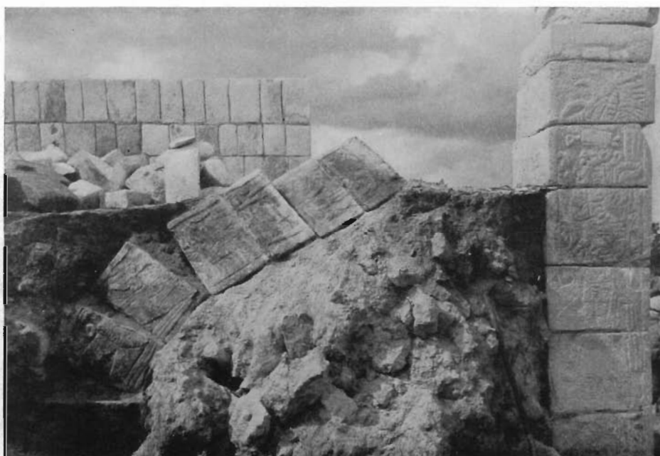
FIG. 67—COLUMN 13, SHOWING DIRECTION OF VAULT FAILURE
